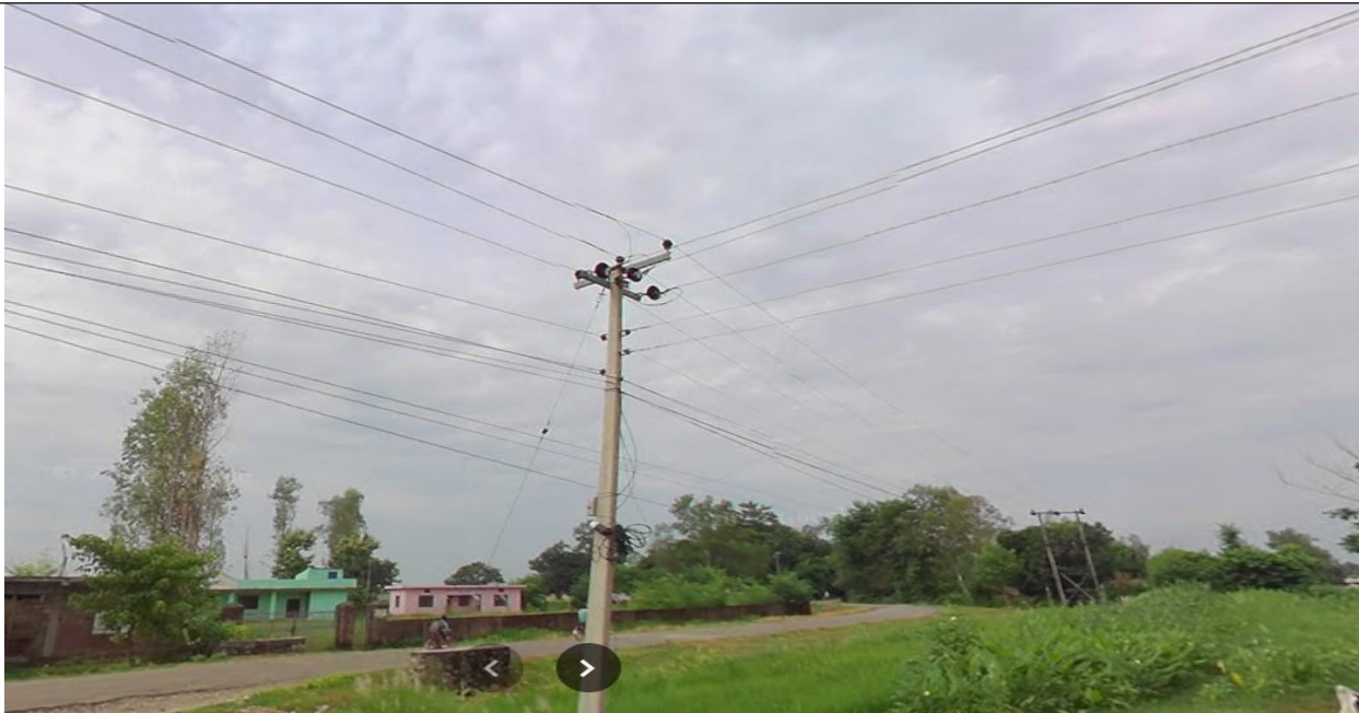
6. 11kVA hightension line just infont of Simarana WSP gate.
